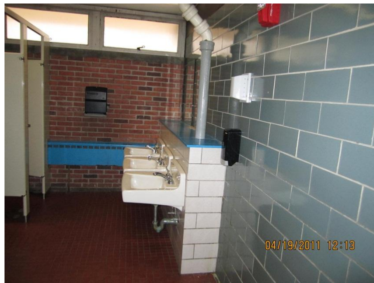
Typical Bathroom Fixtures
