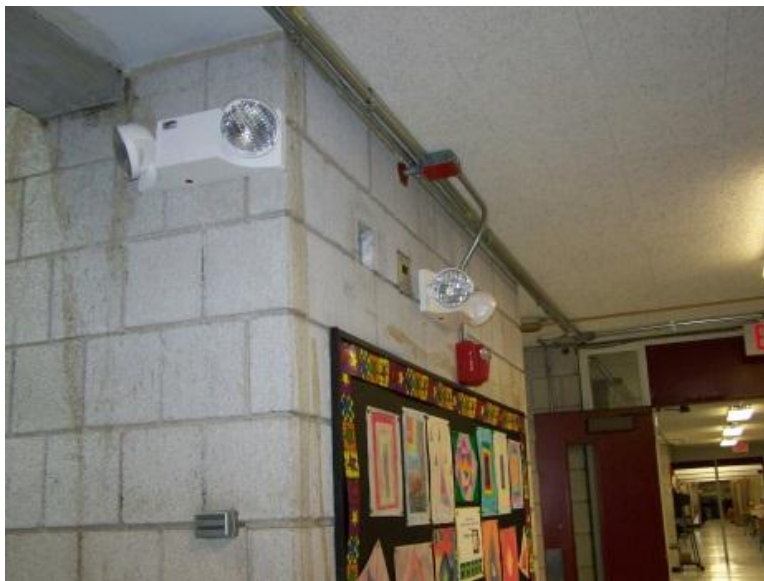
Typical Egress Lighting and Exit Signs
