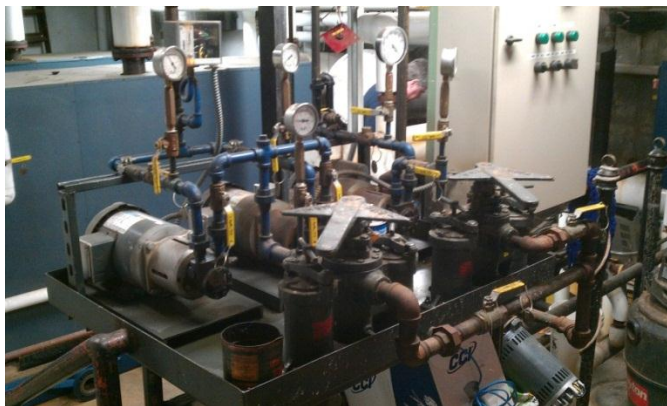
Fuel Oil Pumps
