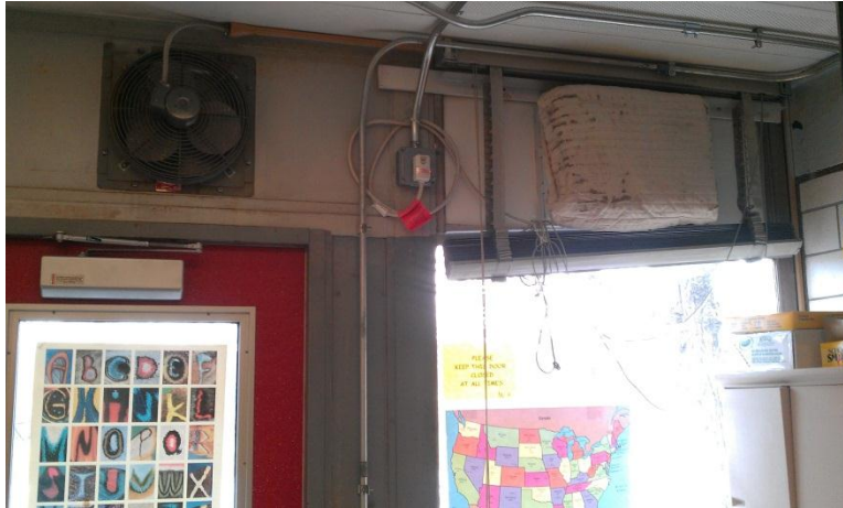
Window Air Conditioning Unit & Wall Exhauster
