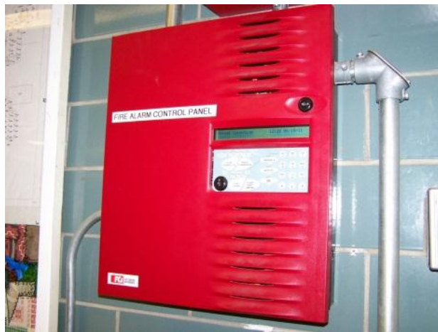
Main Fire Alarm Control Panel
