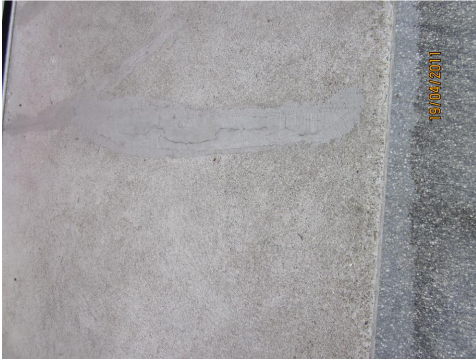
Photo 1: localized cracking at exterior cantilevered slabs on grade.
