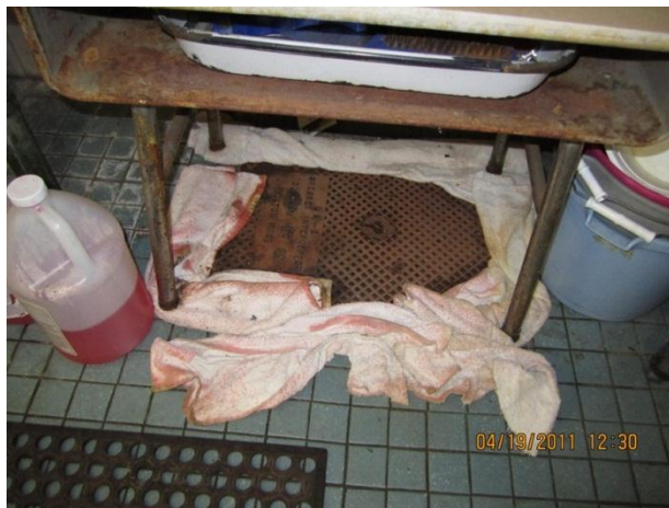
Kitchen Grease Interceptor, Aged and Failing
