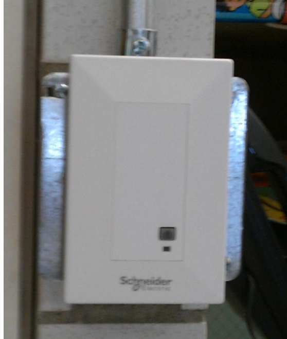
Newer DDC Wall Sensor
