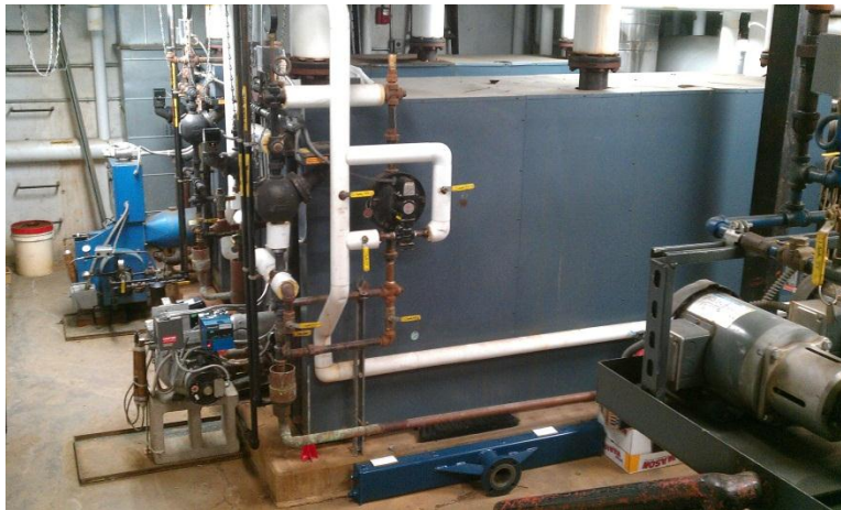
Existing Boilers From 1998 Boiler Room Renovation
