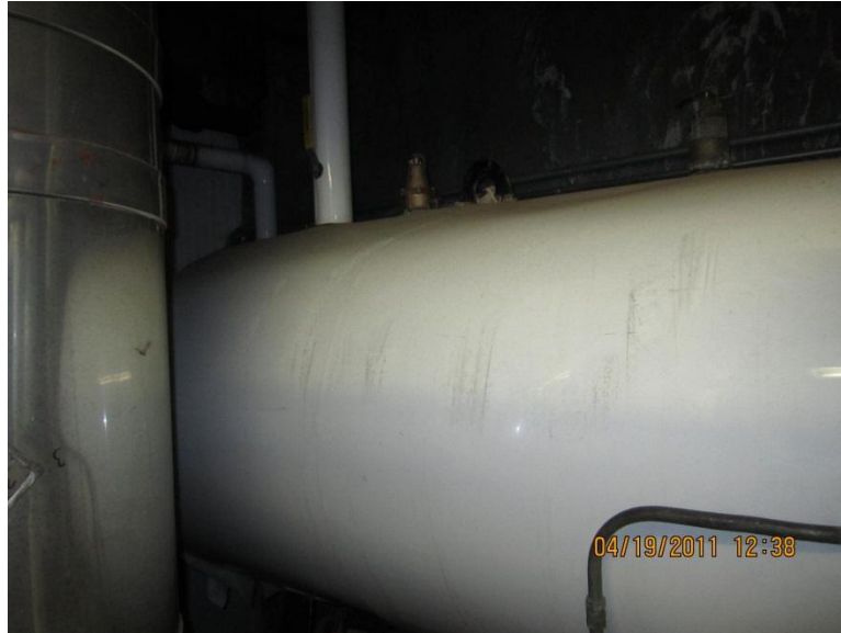
Domestic Hot Water Tank
