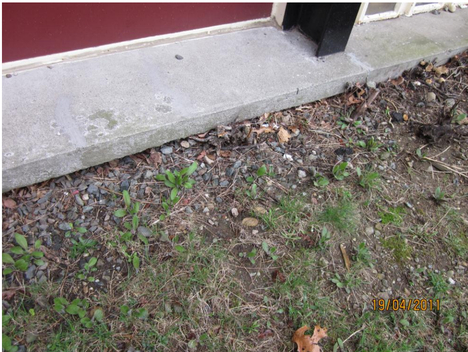
Photo 2: localized cracking at exterior cantilevered slabs on grade.
