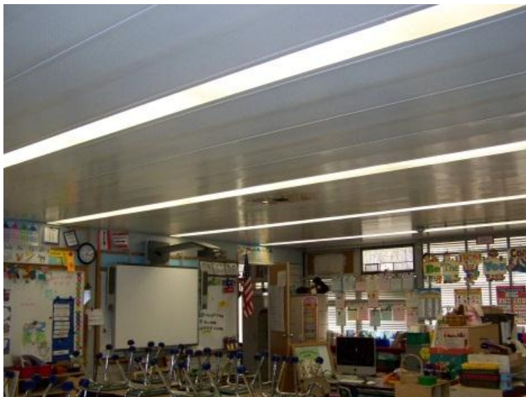
Typical Classroom Fluorescent Fixtures
