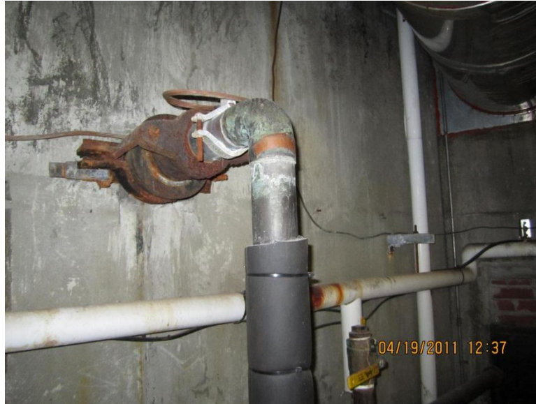
Water Service Entry
