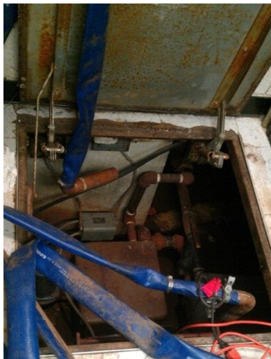
View Into The Underground Trench Where Steam Piping Runs
