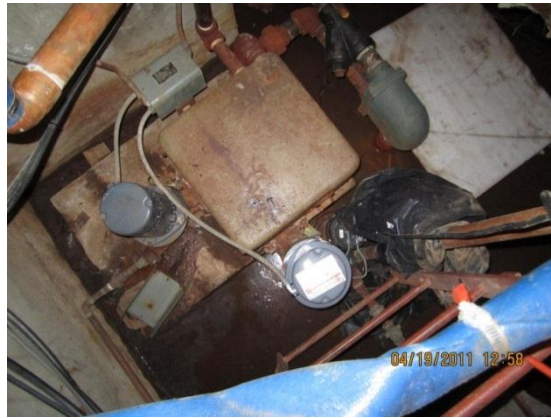
Water In Piping Trench
